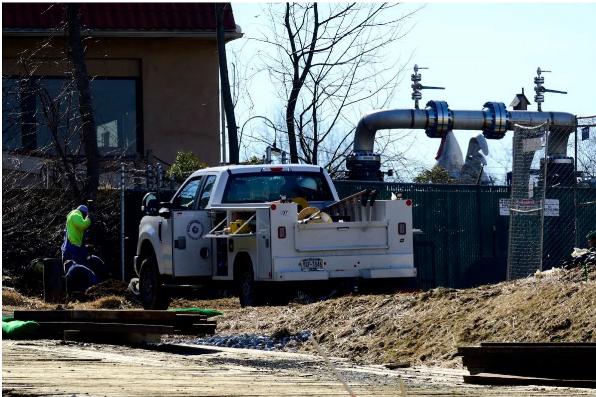
Workers dig near a part of a natural gas liquids pipeline, in West Chester, Pennsylvania, on March 13,
